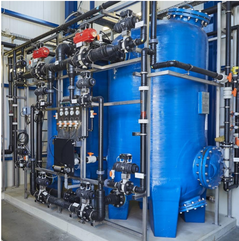
Figure 2. GEH adsorption system with FRP-vessels
